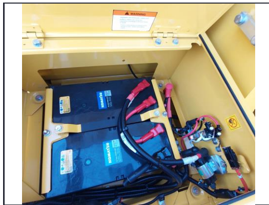
Affixed warning decals installed.
