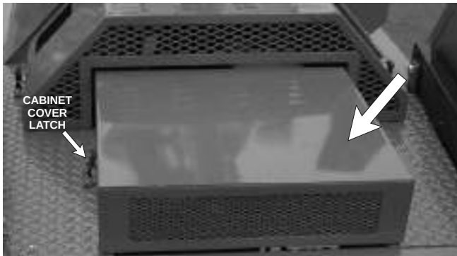
Figure 13.6 - DC Motor Battery Cabinet
